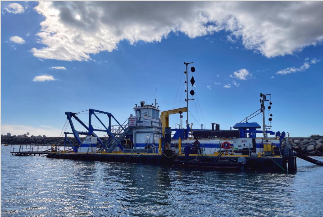
Pictured above the District's dredge, Twin Lakes , as the crew works hard to deepen the channel.
